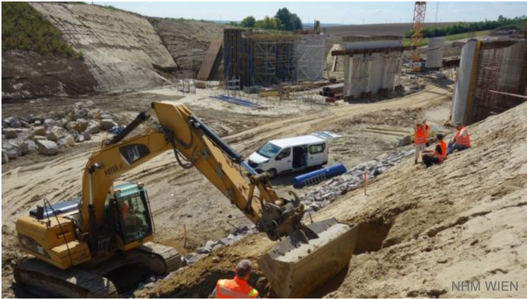
A new road is being built at the site north of Vienna
